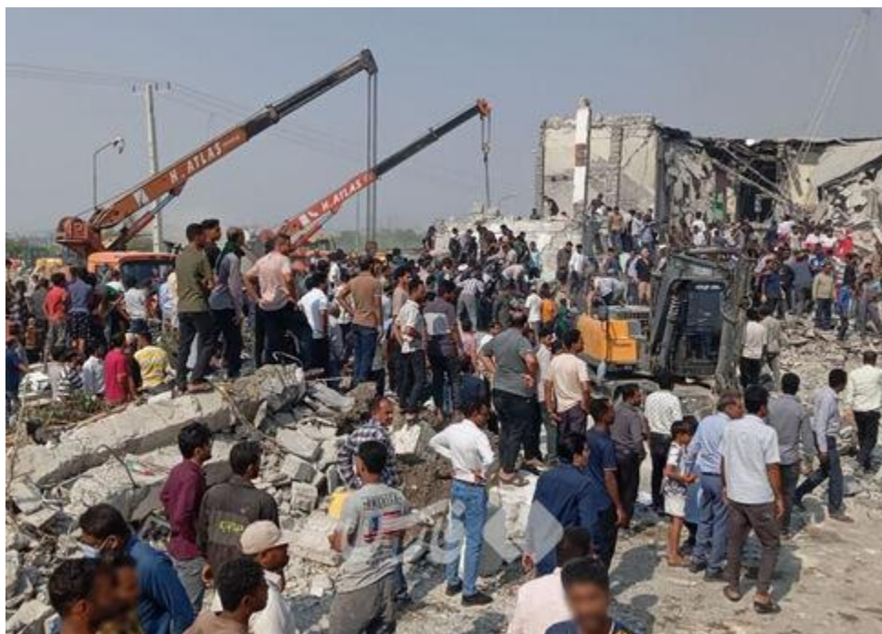
Aftermath of school strike. The distinctive pancaking of the roof is evidence of a top-down air strike which destroyed much of the school building © Private
