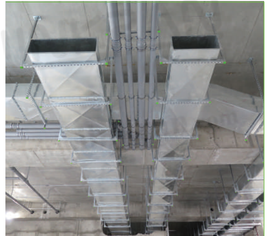
LINKRAN Modular Support Systems Implemented Samples
